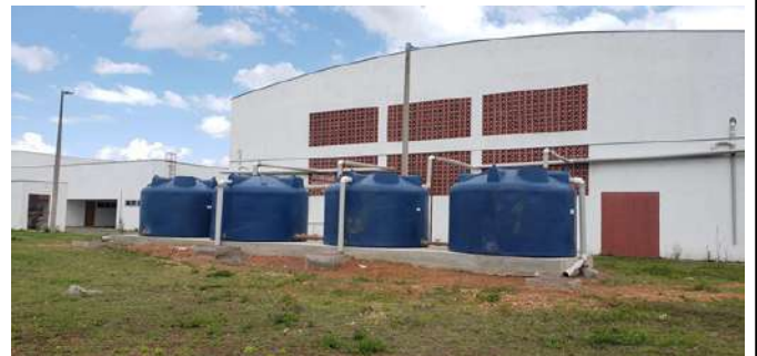
Figure 20: Poços de Caldas Campus rainwater reservoir tanks.
