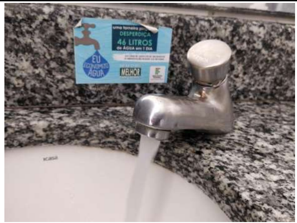
Figure 6: Campus Machado tap with faucet aerator.
