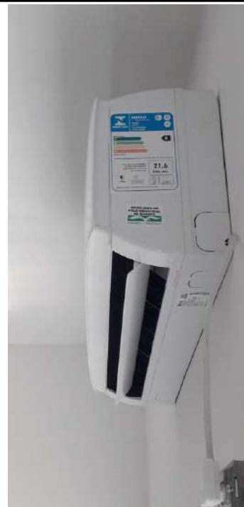
Figure 6: Campus Carmo de Minas efficient air conditioning.
