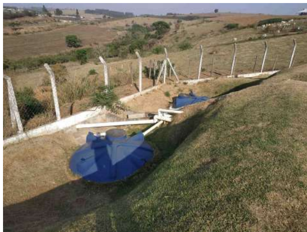
Figure 7: Muzambinho Campus rainwater reservoir tanks.
