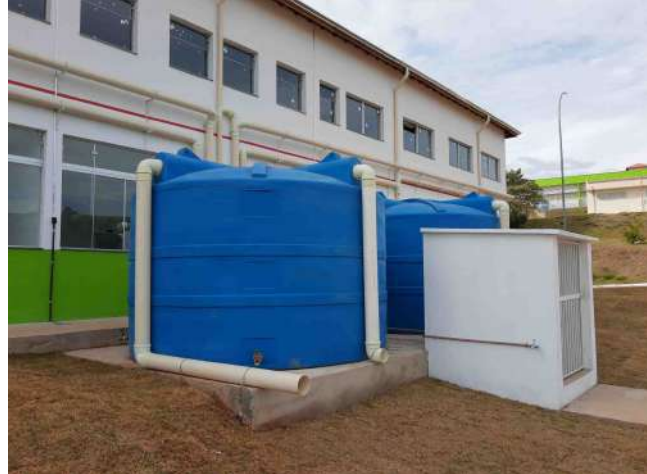
Figure 10: Pouso Alegre Campus rainwater reservoir tanks.
