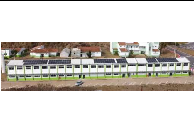
Figure 21 : Campus Machado expansion of the photovoltaic plant.
