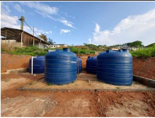
Figure 23: Machado Campus rainwater catchment system for swine sector cleaning.
