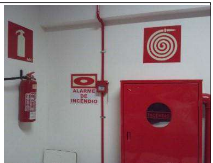
Figure 1: Campus Passos fire-fighting system – Fire extinguisher, fire hose and fire alarm.
