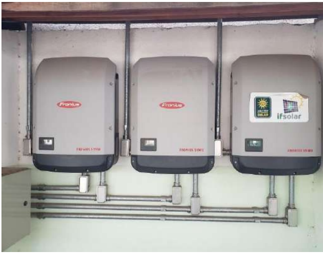
Figure 5: Rectory automatic management system for energy supplies and production – Solar power converters.
