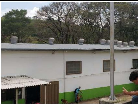
Figure 15: Campus Machado Coffee Roasting Building exhausters.
