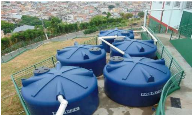
Figure 7: Campus Três Corações rainwater recovery system for covering the flushing and irrigation – Water storage tanks.
