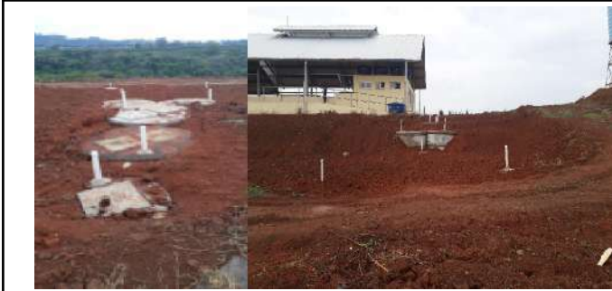
Figure 5: Muzambinho Campus waste treatment.
