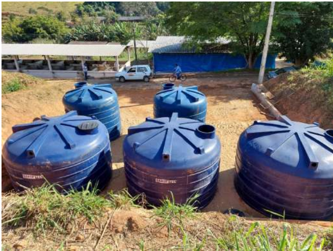
Figure 17: Machado Campus new rainwater reservoir tanks.
