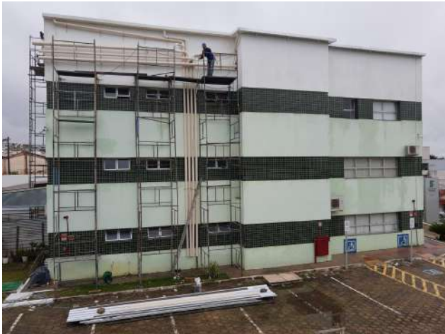
Figure 19: Rectory new rain harvesting system.
