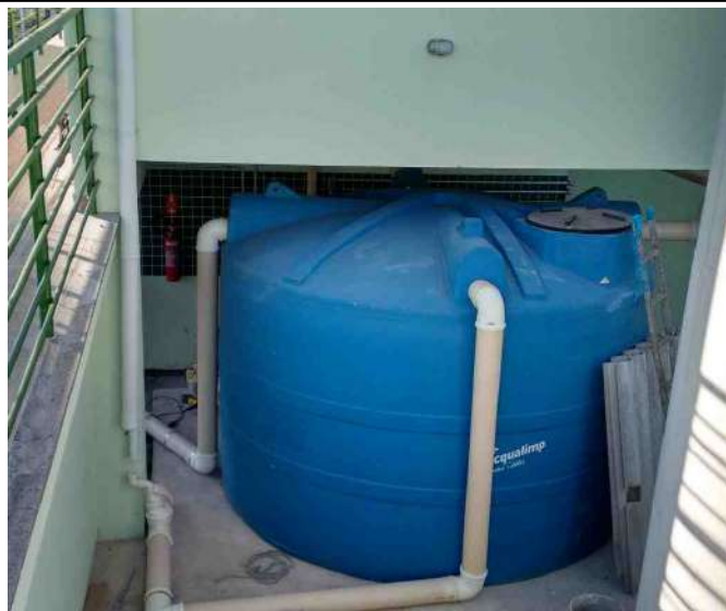
Figure 11: Rectory rainwater reservoir tank.
