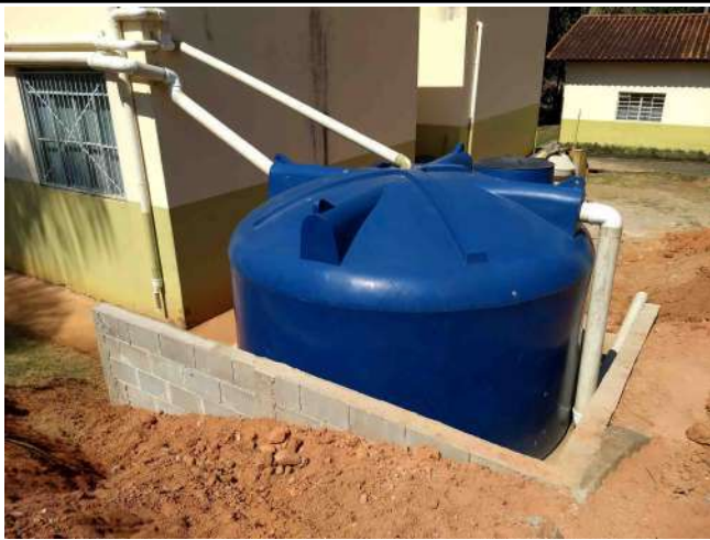
Figure 5: Inconfidentes Campus rainwater reservoir tank.
