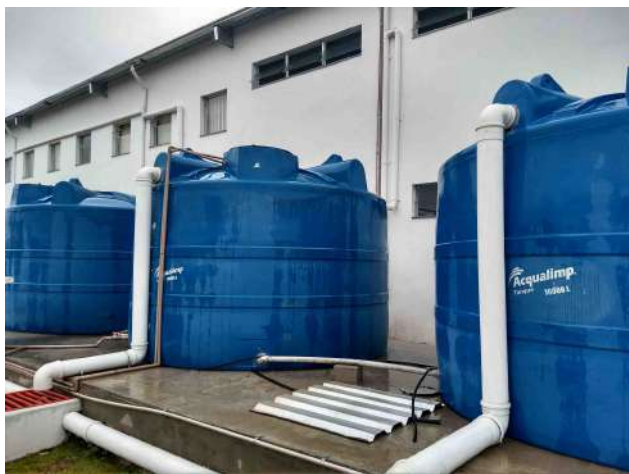
Figure 9: Poços de Caldas Campus rainwater reservoir tanks.
