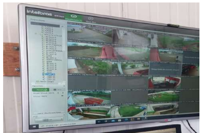
Figure 4: Pouso Alegre Campus CCTV.
