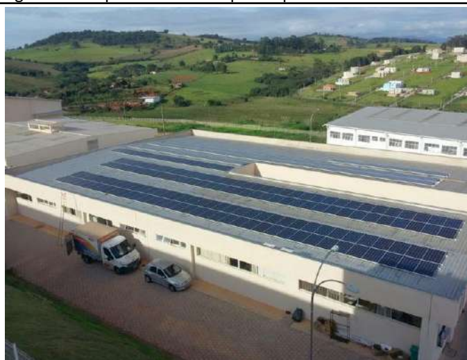
Figure 6: Campus Pouso Alegre solar power plant.
