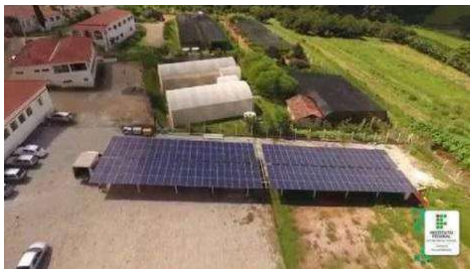
Figure 3: Campus Muzambinho solar power plant.
