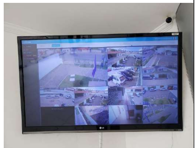
Figure 4: Rectory video surveillance system – Camera control.
