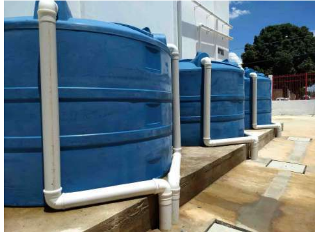
Figure 8: Passos Campus rainwater reservoir tanks.
