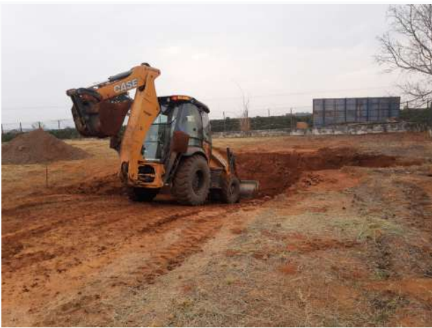
Figure 19: Machado Campus implementation of the Sewage treatment system of the Coffee Center of Excellence.
