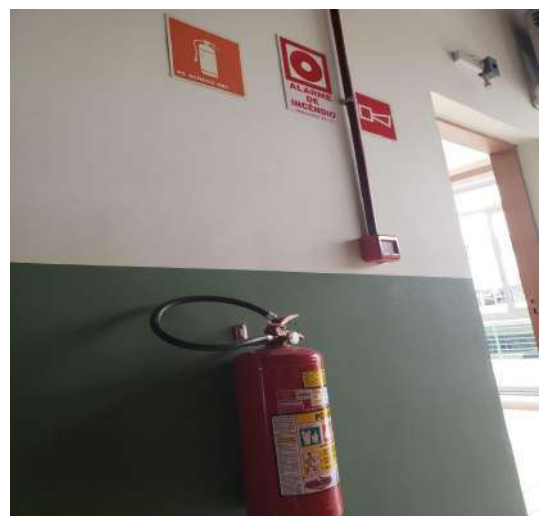
Figure 10: Rectory fire alarm and fire extinguisher.
