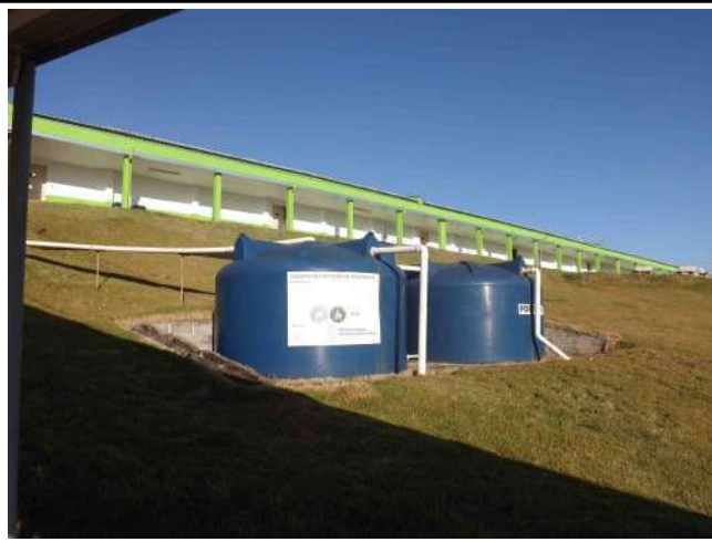
Figure 6: Machado Campus rainwater reservoir tanks.
