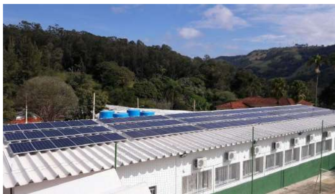
Figure 7: Campus Carmo de Minas solar power plant.
