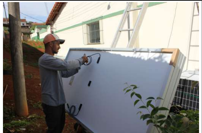
Figure 22: Inconfidentes Campus expansion of the solar power plant.
