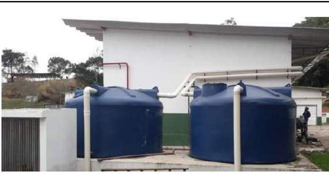
Figure 13: Carmo de Minas Campus rainwater reservoir tanks.
