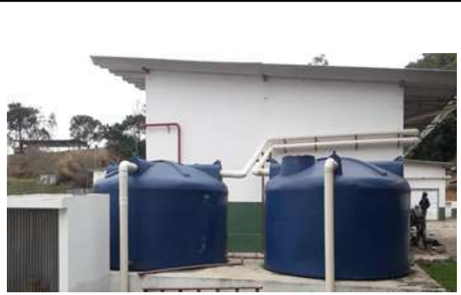
Figure 24: Carmo de Minas Campus rainwater catchment system
