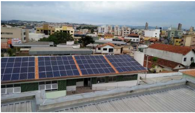
Figure 9: Rectory solar power plant.
