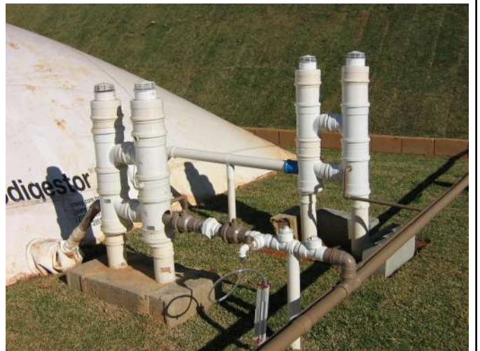
Figure 14. Swine waste treatment unit for biogas production.
