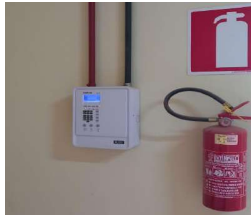
Figure 8: Pouso Alegre fire alarm and fire extinguisher.
