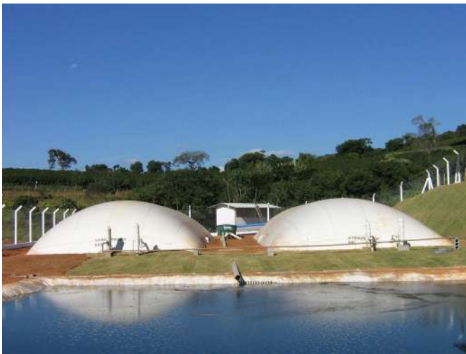
Figure 13. Swine waste treatment unit for biogas production.
