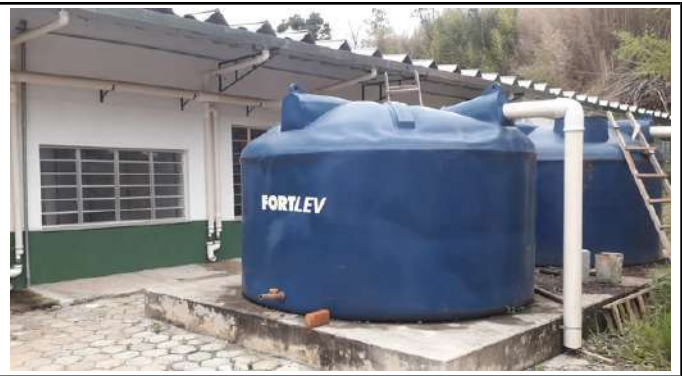
Figure 14: Carmo de Minas Campus rain harvesting system.
