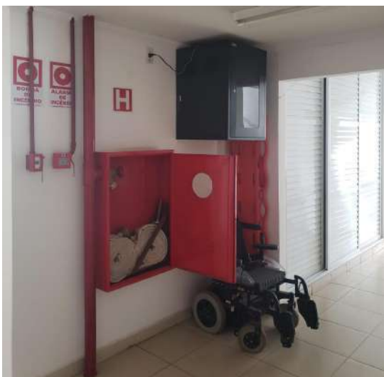
Figure 9: Rectory fire alarm and hydrant.
